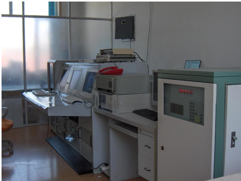
Figure 3. Changchun SLR & LTT Control Room
